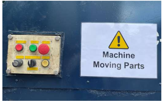
Figure 6: Visible signage that warns of moving parts
